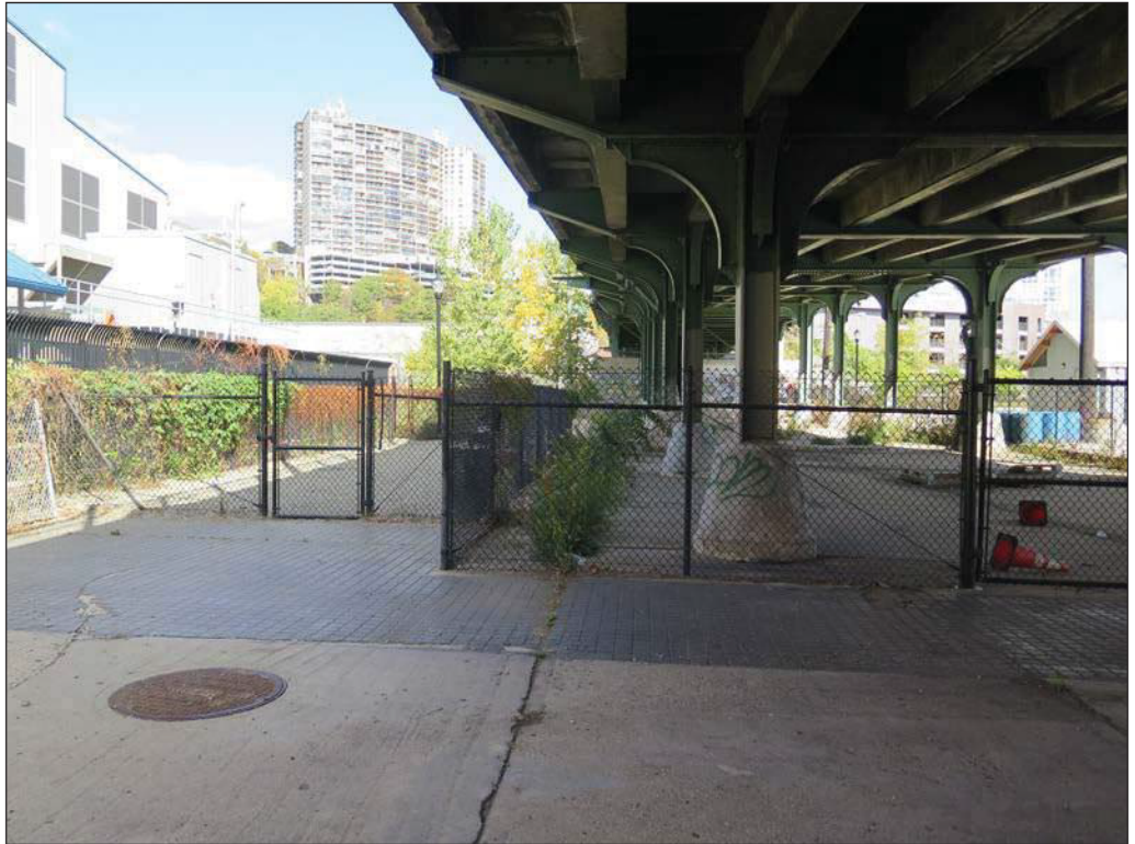
View north of the potential underpinning location at the Willow Avenue Bridge. 11
